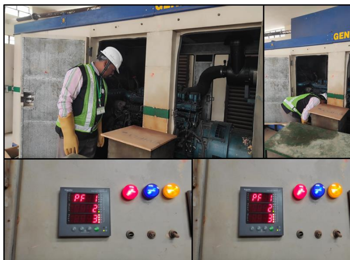
Energy conservation facilities observed in the Campus
