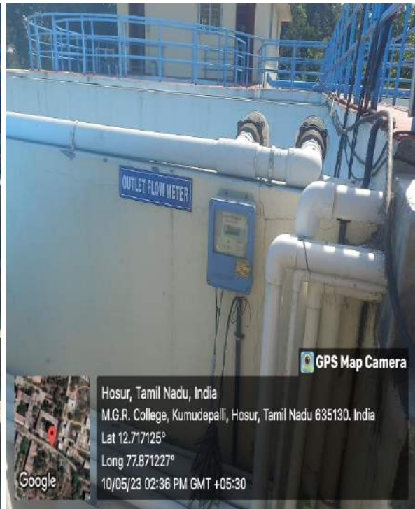
Outlet Flow Meter
