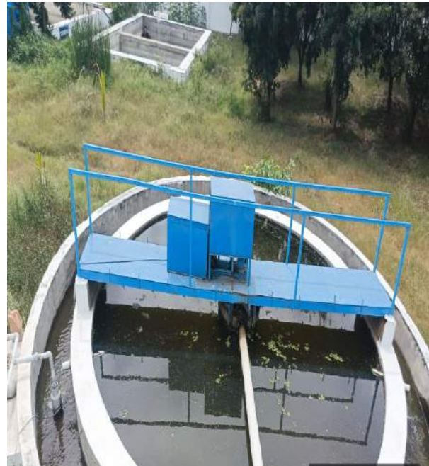
Sewage Treatment Plant
