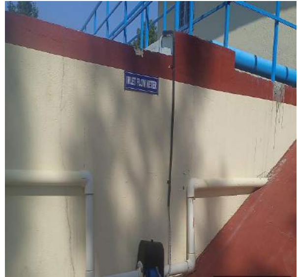
Inlet Flow Meter
